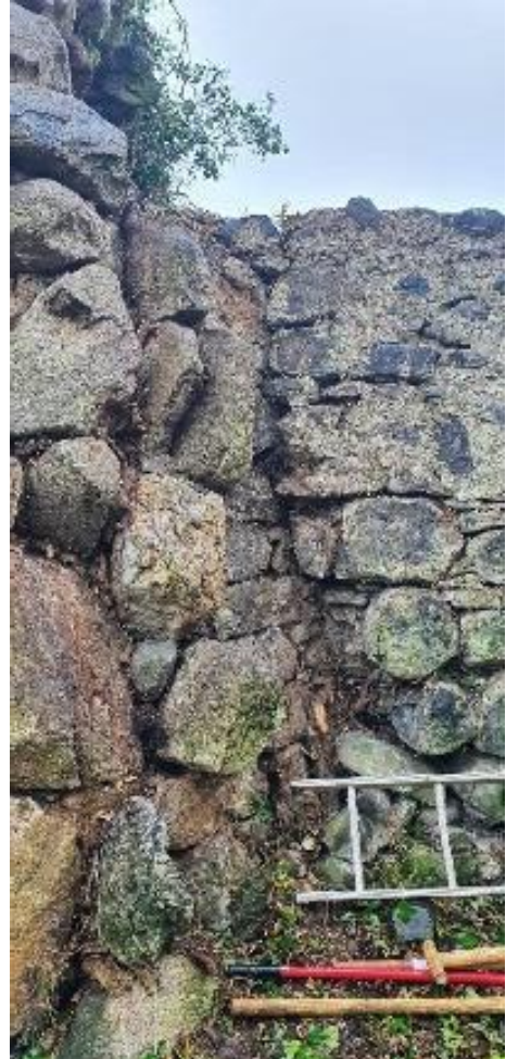
Figure 12 – Stone missing where wall abuts arch
