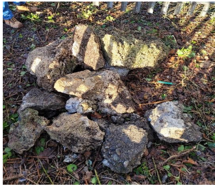
Fallen stones from Arch top lying to North-East of Arch
