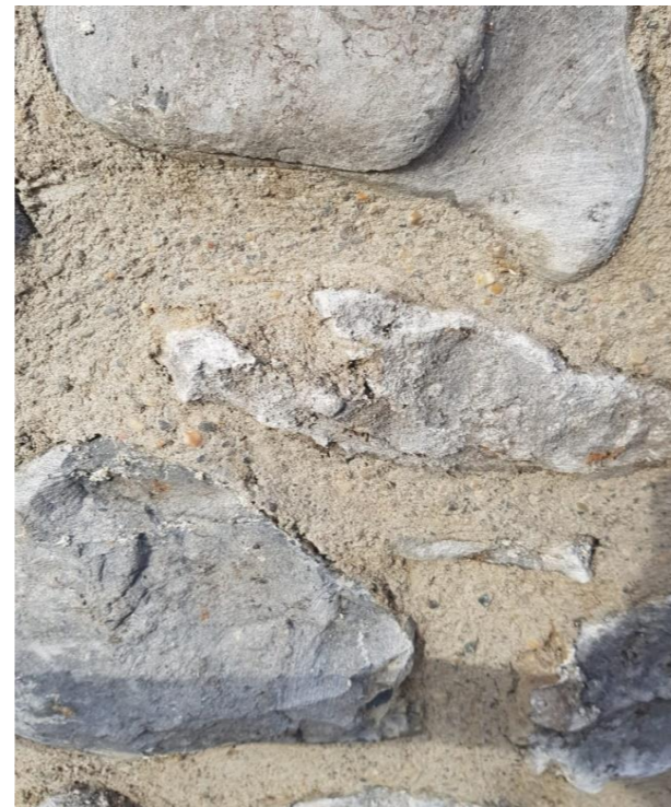
Exemplar provided of flush pointing in stonework beaten back to expose aggregate
