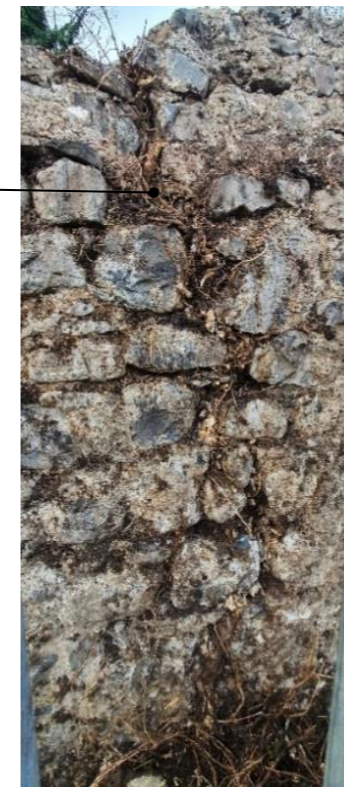
Outer face of South-East Flanking Wall showing vertical cracks
